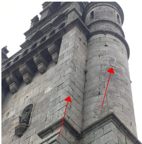
Clocher - Joints creux
